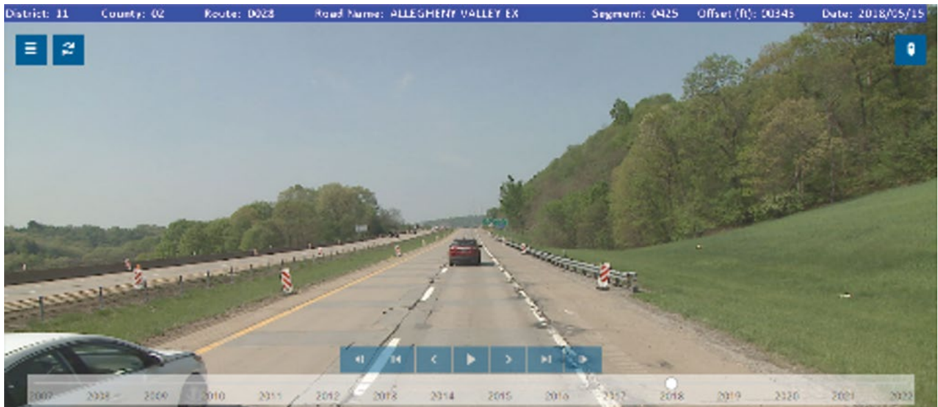
Figure 6.6 Surface Conditions of SR-28, Section A55 in Allegheny County in 2018 Before Rehabilitation (Courtesy of PennDOT)
