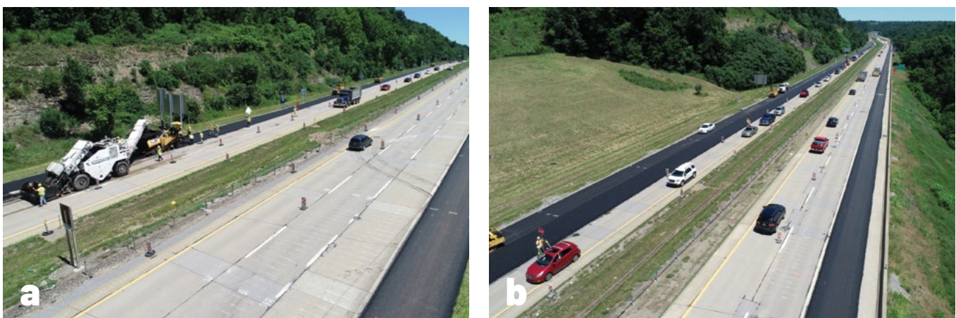
Figure 6.10 Construction of Asphalt Overlay over B&S JRCP: a) Paving Exit Ramp, and b) Paving Main Lane (Courtesy of PennDOT)
