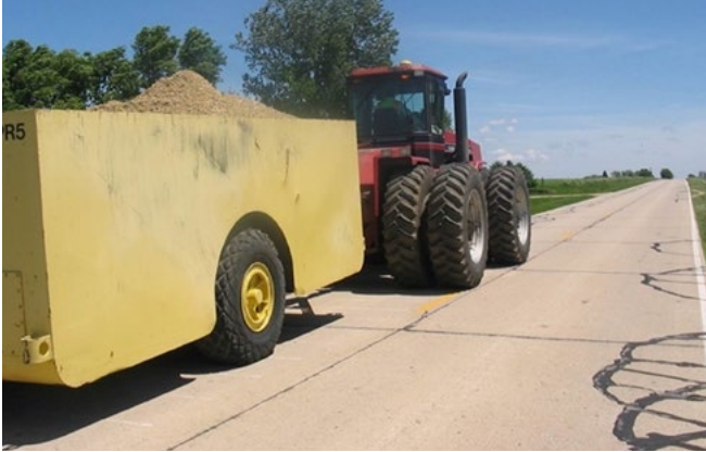
a. Seating after Cracking
