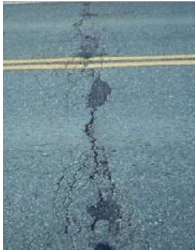
Figure 2.4 Deteriorated Reflection Crack Area (NAPA 1999)
