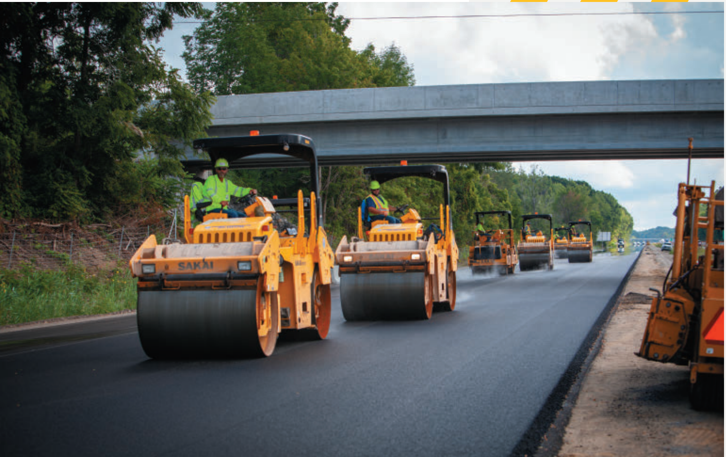
Lindy Paving crews roll down I-90 during work that earned the company its record sixth Sheldon G. Hayes Award. (See page 28)
