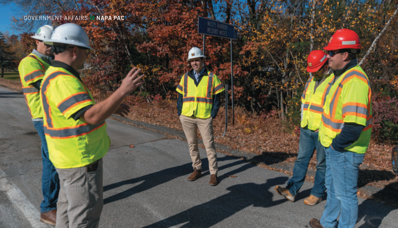
Rep. Chris Pappas (D-NH) meets with Pike Industries personnel at a job site.
